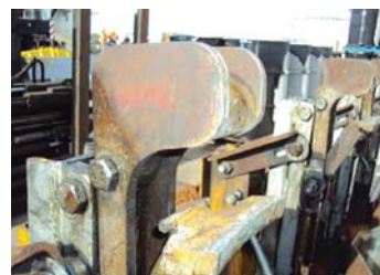
Handling gear equipment to transport drums
