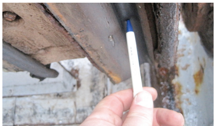
Ascertaining deformation on hatch sealing
